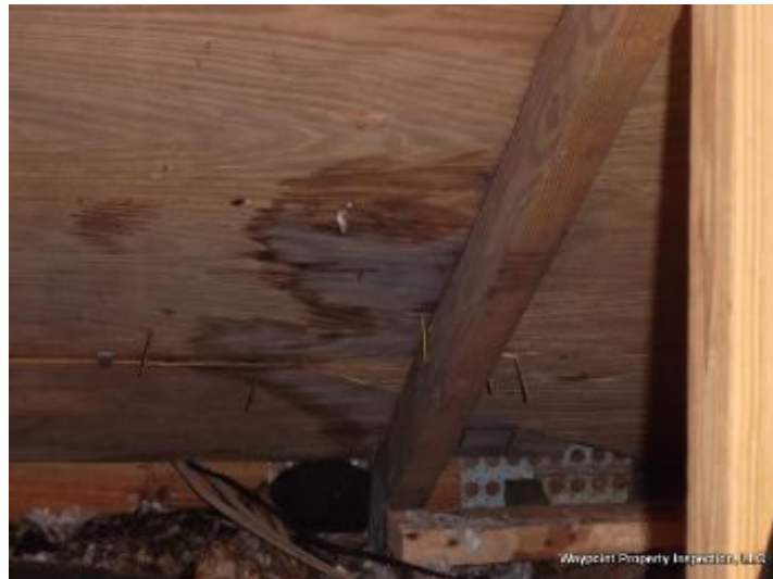
Moderate stains/damage visible at South hallway. Tested wet. Suggest evaluation and repair.
