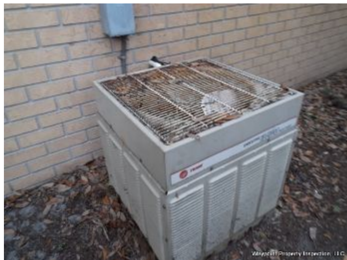
Cooling system 1 has surpassed its manufacturer's life expectancy (12 - 15 years.) Suggest full evaluation by a qualified HVAC specialist.
