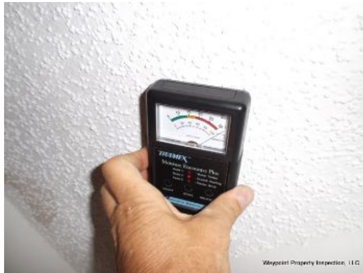
Moisture detected at South hallway. See attic notes.
