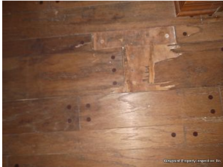
Damage visible at wood flooring.
