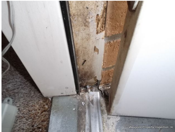
Moisture and WDO like damage visible at secondary door(s) jamb. Recommend evaluation by WDO licensed tradesman.
