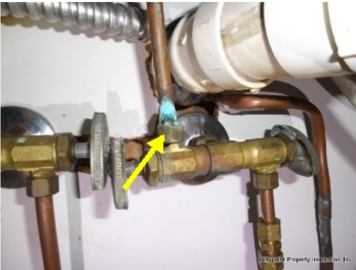
Pipes under kitchen sink are corroded.
