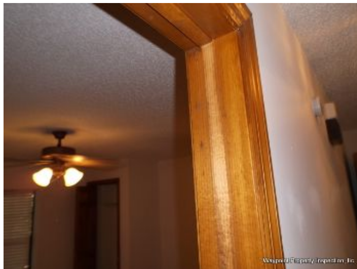
Missing trim at secondary bedroom.
