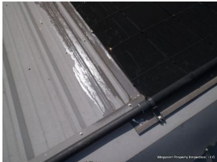
Solar panels are leaking.
