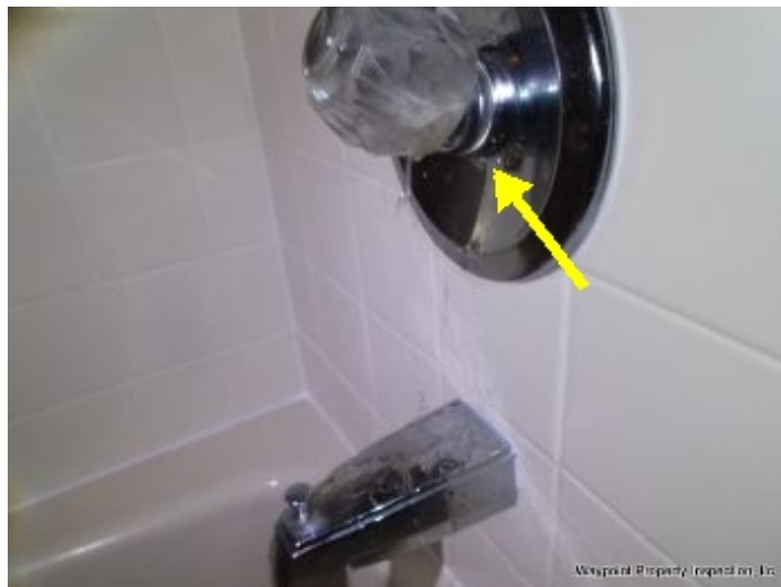
Faucet control leaks at master bathroom.
